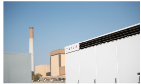
Tesla battery located at Rawhide Energy Station
