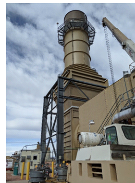
Natural gas combustion turbine unit F at Rawhide Energy Station.
