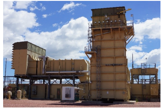
Natural gas combustion turbine at Rawhide Energy Station.
