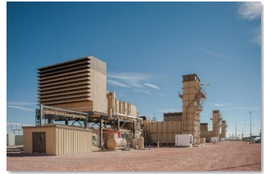
Combustion Turbines at Rawhide Energy Station
